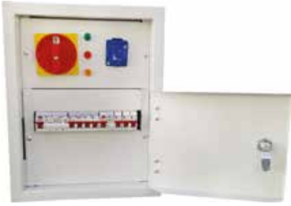
Elektrik Panosu / Electricity Panel
